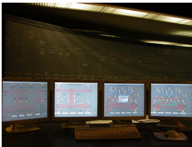
Fig. 1 – Control position of the SCTE system at RFI Firenze Campo di Marte
